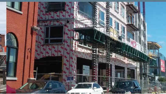
(Clockwise from left) Earlier this year portions of the former Portland Company complex not protected by the new historic district were demolished; The India Street neighborhood has seen rapid development like this new building at 20 Thames Street; Preserving Landmarks like John Ford's home on Munjoy Hill have been at the forefront of Landmarks' advocacy this year.
